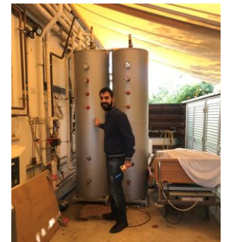
Photos of the hospital's boilers
